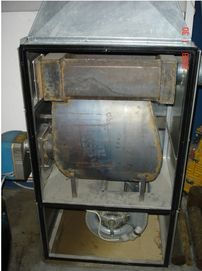
Figure 3 Exposed heat exchanger surfaces of the 30,000 kcal / h air furnace, after the removal the front cover and the fan inlet grid.
